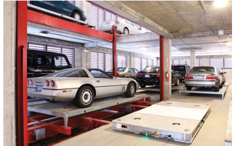
FIGURE 105 - BOOMERANG ROBOTIC PARKING SYSTEM
